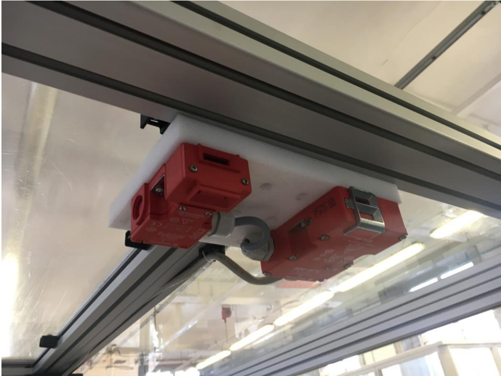
Figure 4: Safety switches fitted to the enclosure
